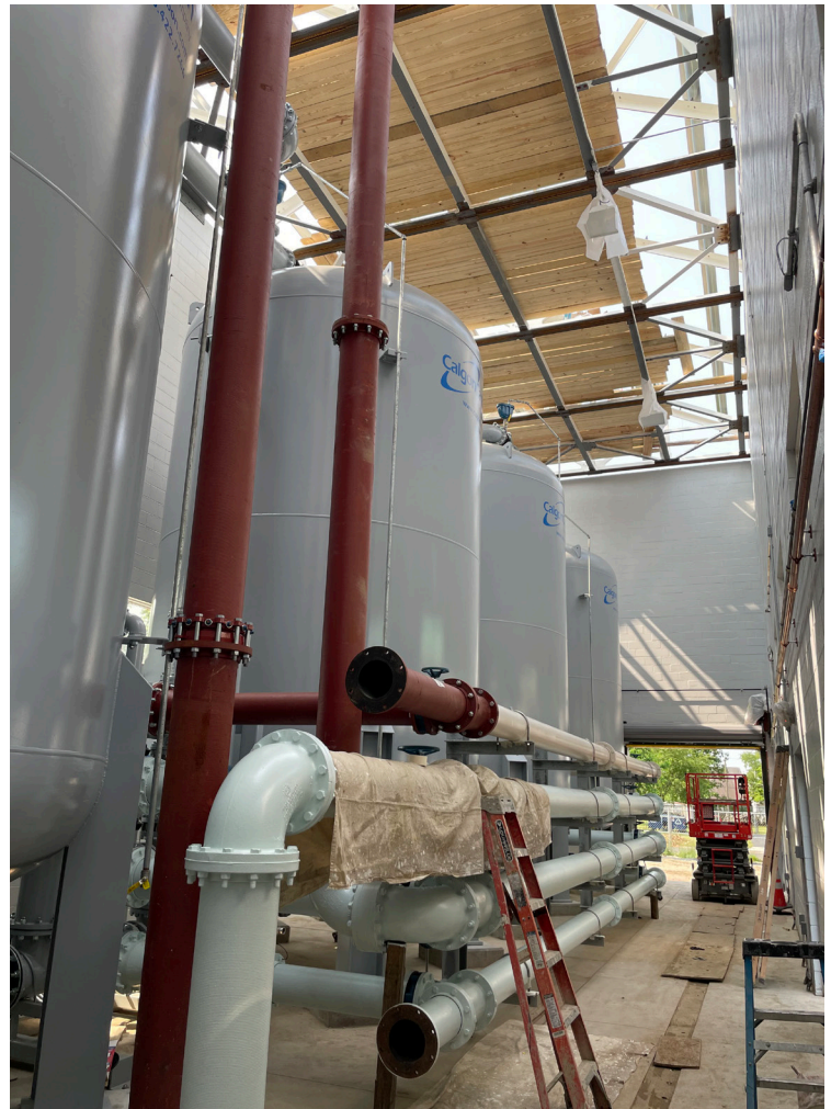
New GAC Treatment Equipment at Willingboro
