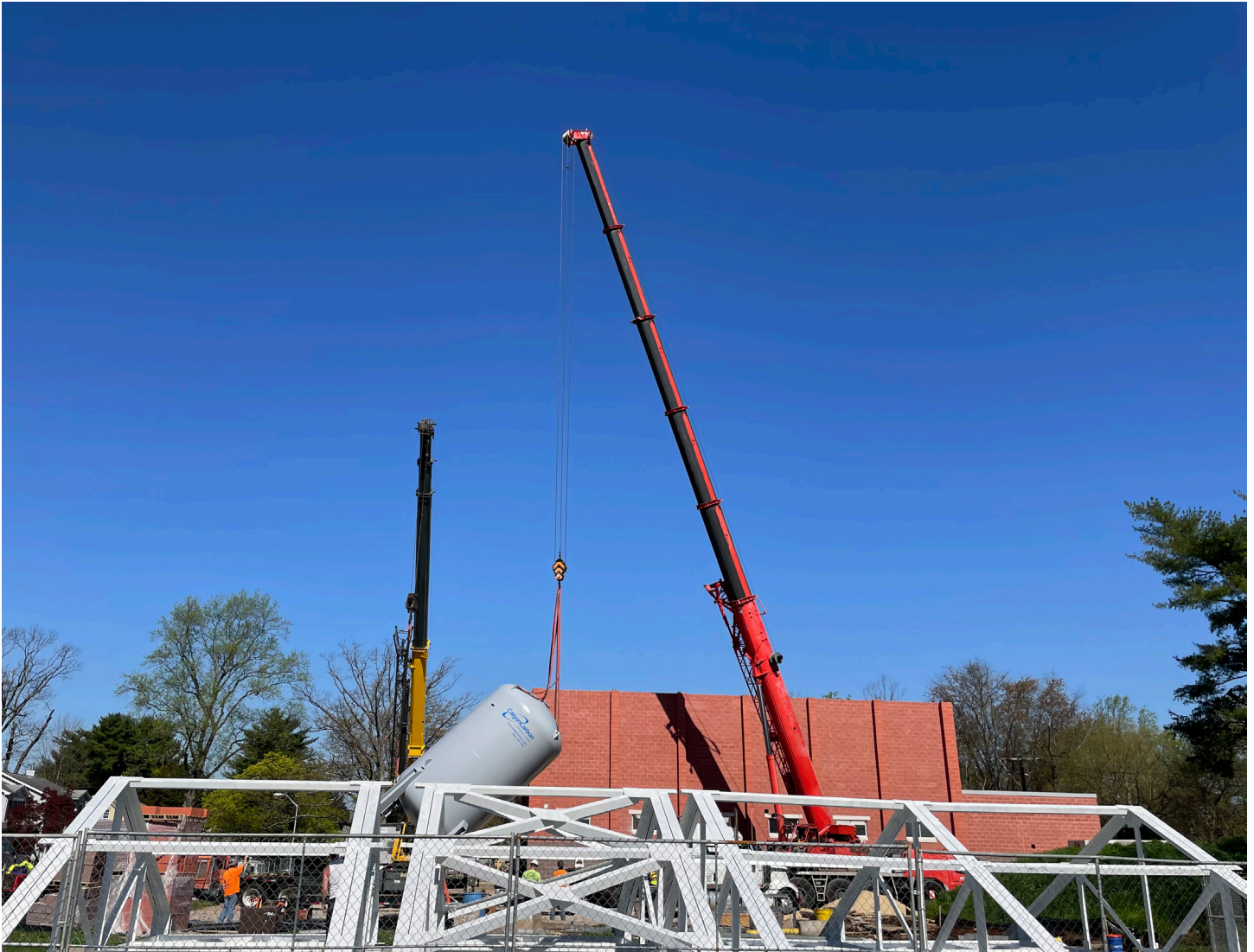
Willingboro PFAS treatment Installation
